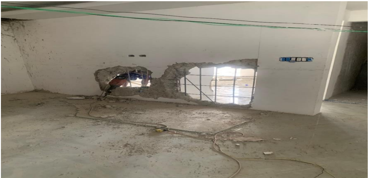
Figure 2 depicting the demolition of an additional concrete wall in the living/dining area on the ground floor
