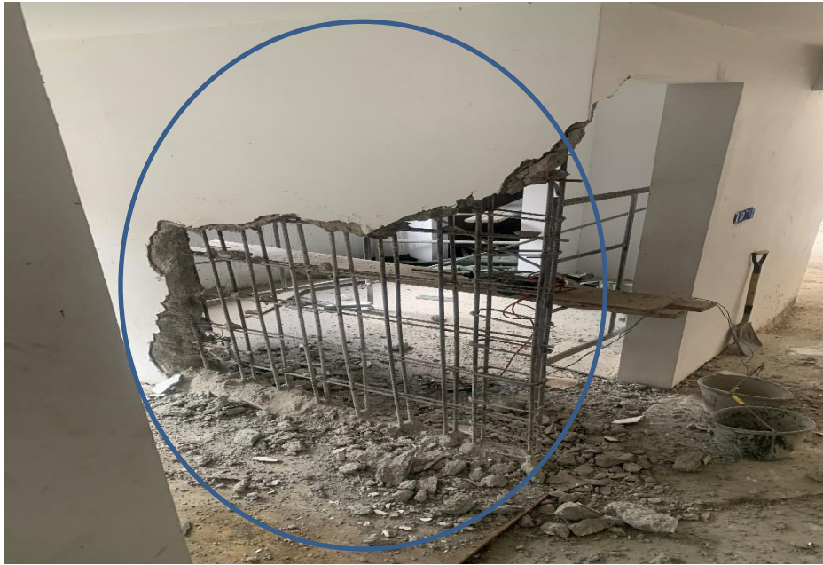
Appendix #1 – Demolition of Concrete partition wall in Laundry Room at Split Level.
