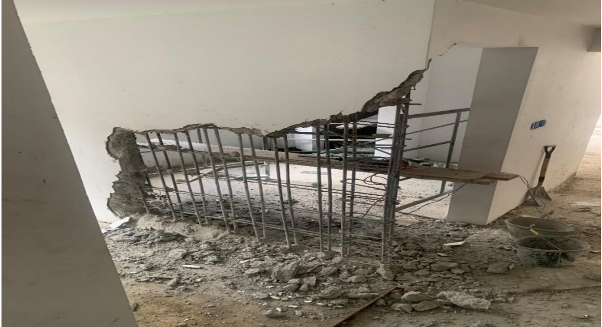
Figure 1 depicting the demolition of an additional concrete partition wall in the laundry room at split level.
