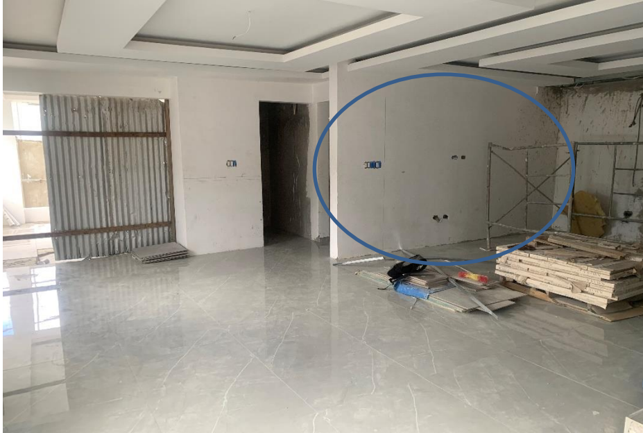
Appendix #2 – Additional concrete wall on Ground Floor, with electrical, painting and tiling works ongoing.
