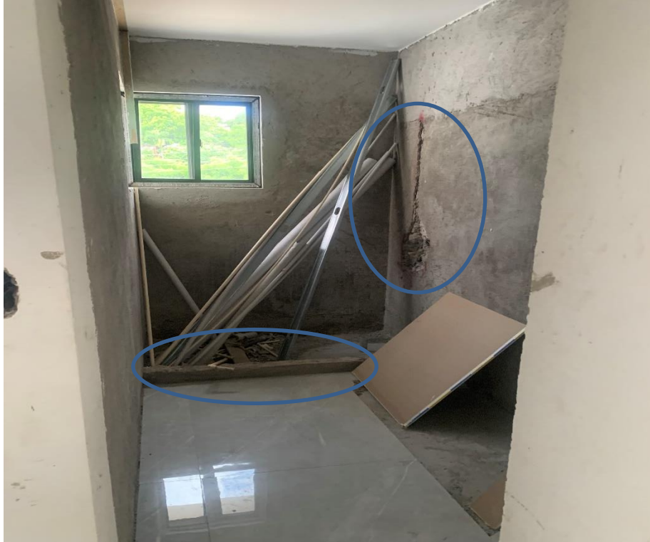
Appendix #6 – Additional en suite bathroom on first floor with standing shower toe wall constructed and provision for plumbing works ongoing.
